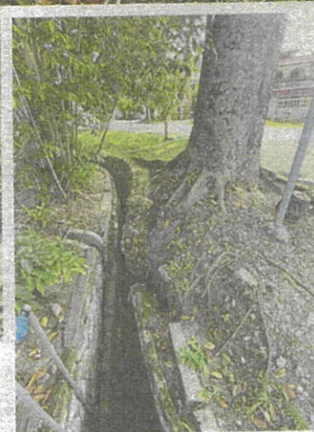
The two trees felled at Jalan Tanjung 12 in Taman Seputeh, Kuala Lumpur. (Inset) Protruding roots of a mahogany tree along Jalan Taman Seputeh have caused cracks in the drain structure.
