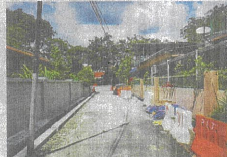
The damaged drain in Jalan Sampadi, Taman Setapak was rectified by DBKL last month.
