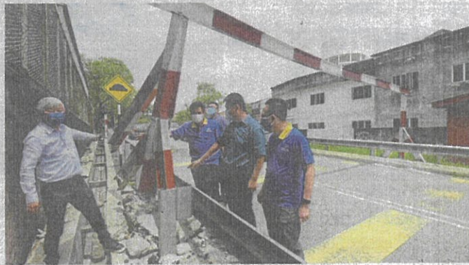
(From left) Puchong MCA new media bureau chief Soon Mon Huay, Liew, complaints bureau chief Wong Jung Lik and government monitoring bureau chief Dr Wong Kok Fye inspecting the damaged height barrier along Jalan Jinma 7 in Seri Kembangan.
