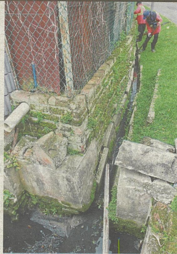
The drains in Jinjang Selatan are too shallow and cannot cope with the amount of water, especially after a downpour.
