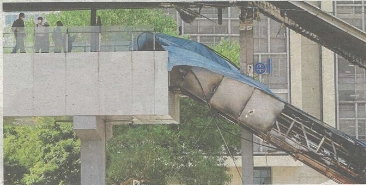
Intermark Mall says it will provide regular updates on the link bridge access and replacement of the escalator which caught fire. — SAMUEL ONG/The Star
