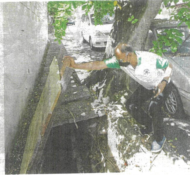
Ganesan looking at a drain that has been damaged by tree roots.
