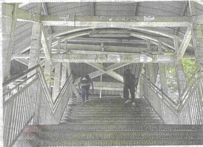
The flooring on this old foot bridge, used by train commuters from Abdullah Hukum and Putra Ria apartments, has worn smooth and the lights are out of order.
