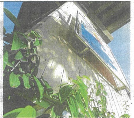
Steel frames installed on Duke 2 pillars to encourage the growth of creepers.
