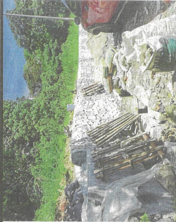
The drainage system along Jalan Kolam Air is being upgraded by DBKL.
