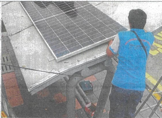
A DBKL contractor installing solar panels on a bus stop's roof in Wangsa Maju.
