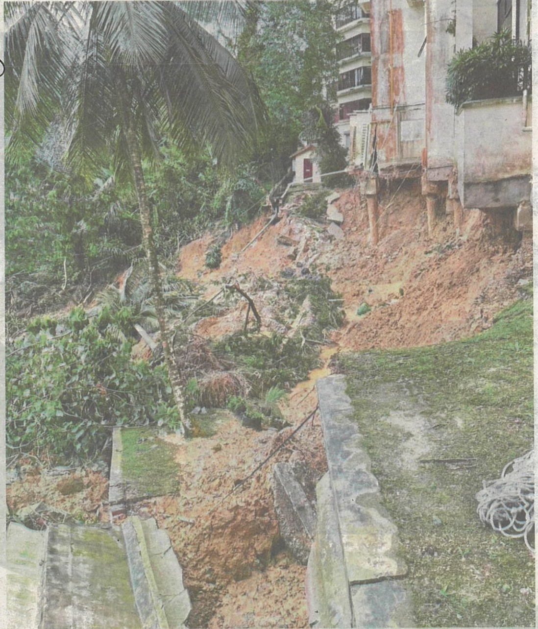
Worrying sight: The precarious situation of Sri Duta 1 condominium in Kuala Lumpur. — Pic from Balai Bomba Sentul's Facebook page
